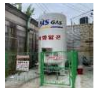
Liquid Storage Tank (L-Ar)
