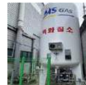
Liquid Storage Tank (L-N2)
