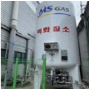
Liquid Storage Tank (L-N2)
