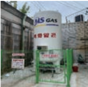
Liquid Storage Tank (L-Ar)
