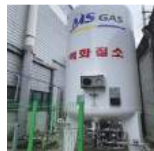
Liquid Storage Tank (L-N2)
