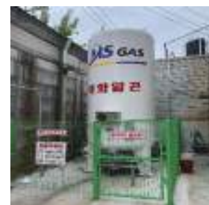
Liquid Storage Tank (L-Ar)
